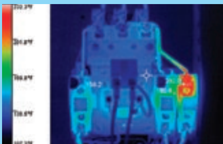
The connections on this evaporator pump read over 50 degrees hotter on phase C.
